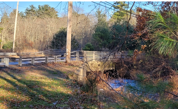
RT. 140 BRIDGE Dam removal will have little impact on water levels + flows at the bridge.
