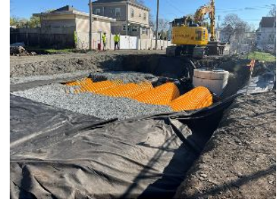
Subsurface infiltration chambers
