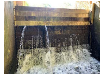
Example of stop logs
