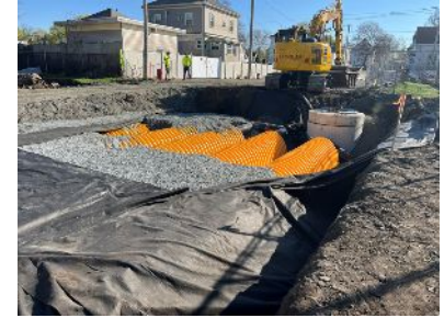
Subsurface infiltration chambers
