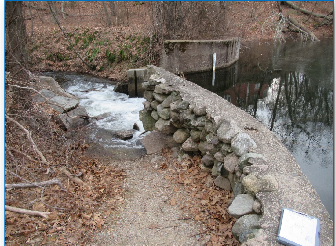
Eroded embankment west of spillway
