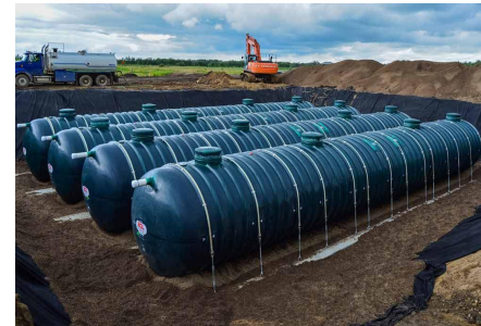
Tank with controlled outlet
