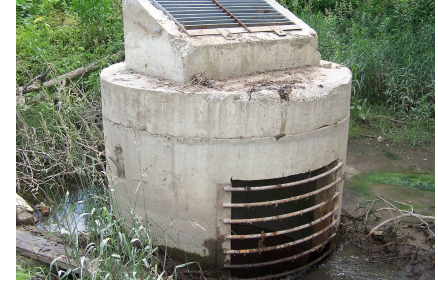
Controlled outlet structure in retention pond
