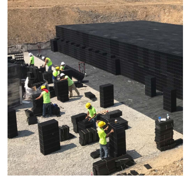
Modular storage with ability to infiltrate
